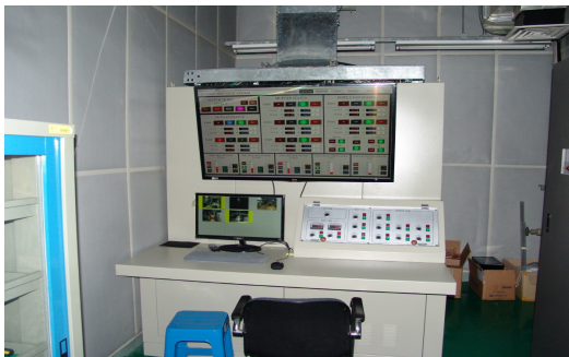
Fig. 2. Newly installed HVAC control panel.
