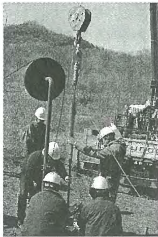
Fig. 2. Field demonstration of straddle packer system
